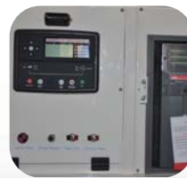
Control Panel & MCB
